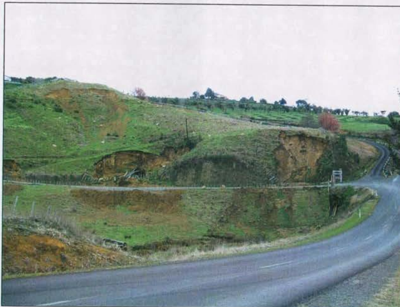
Photo 1: Recent slips adjacent road cut into existing slope following a period of heavy rainfall
