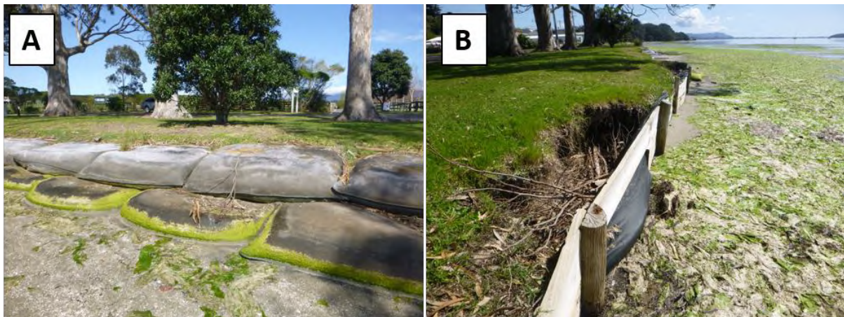
Figure 3-3 Examples of protection structures along the Ongare shoreline. (A) Sandbag seawall (Cell 3C), (B) timber seawall (Cell 3C).
