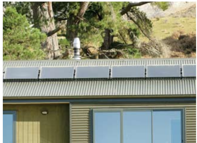
The system uses a Thermocell solar water heater.
