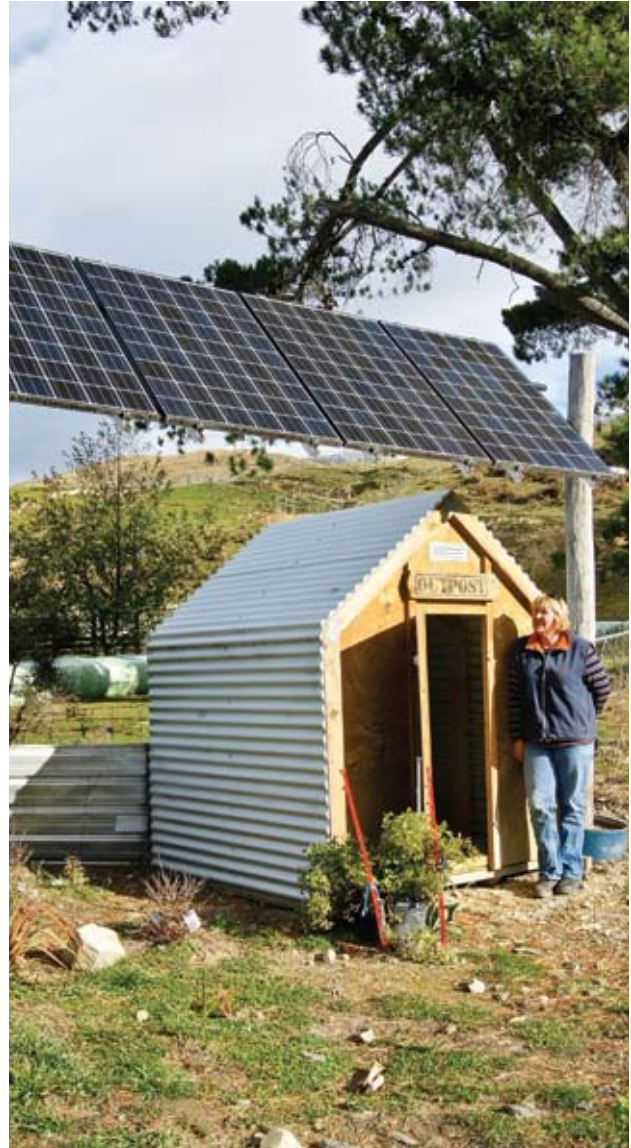
Maree's system has four 200 W photovoltaic modules.
