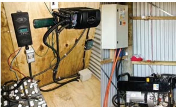
The batteries, controller and inverter are separated from the diesel generator.
