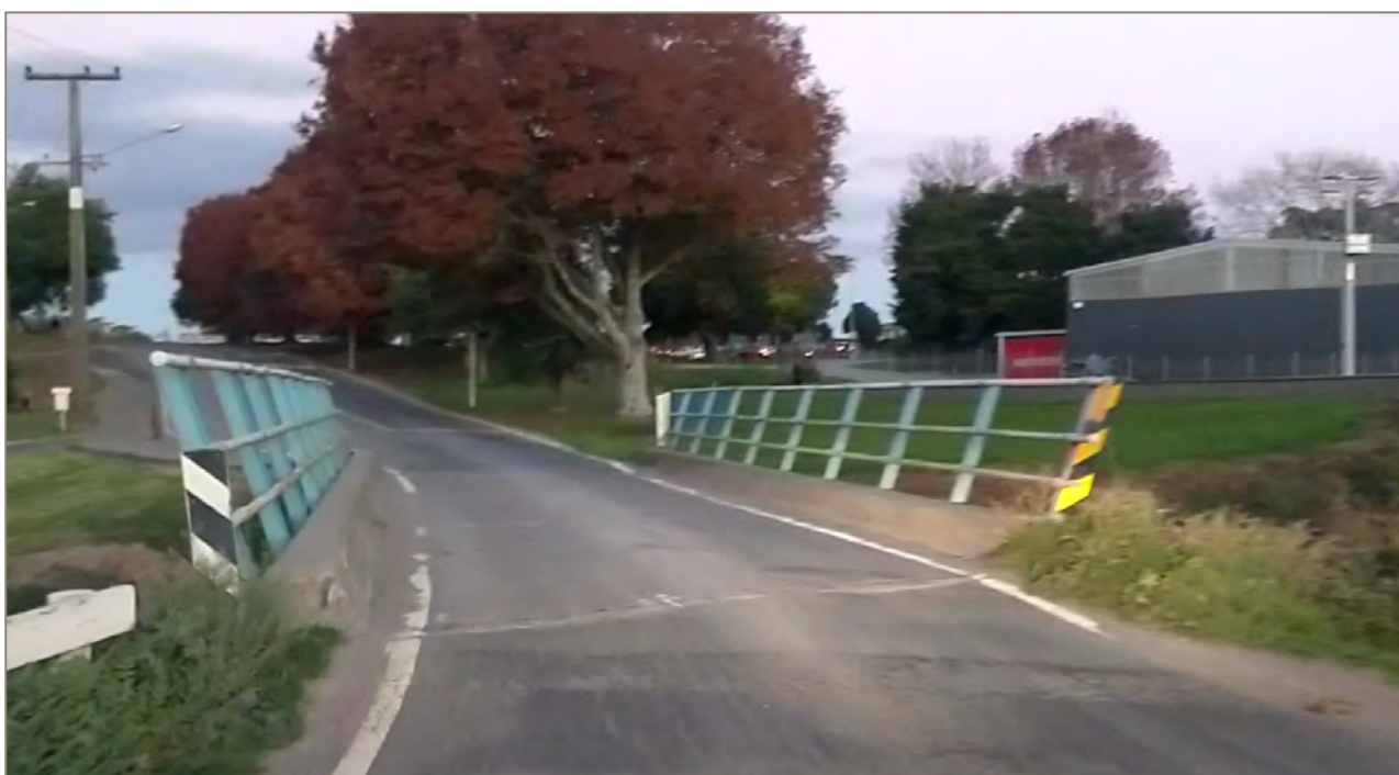
Figure 7-2: Single-Lane Bridge with No Pedestrian Facility
