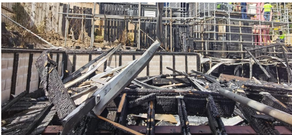
Figure 7: The extent of damage to Dwelling 3 – View from North (entry access way)
