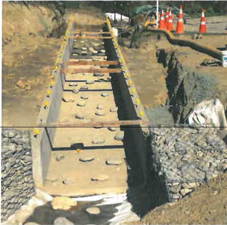
Grouted Rock Baffle Arrangement (Orphanage Stream, Nelson) Reference: Photo by William Dufour (T+T Nelson).
