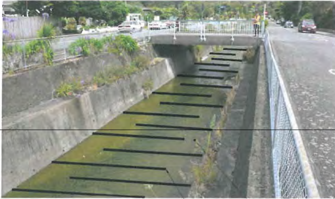
Visualisation of an alternating baffle option in a flat concrete channel. Baffles or alternatively meander deflectors. Materials options include gabions, soil bags, boulders or concrete/shotcrete to create a meander profile. The baffles are intended to trap natural stream bed material.
