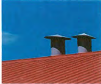
Before: Two outdated extractor fan outlets.
