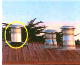
After: 1x new extractor fan (yellow) and two 'upgraded' extractor fan outlets.
