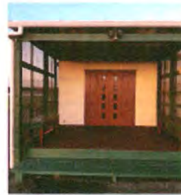
Whare Kai Porch: New drainage, roofing iron and flashings in complimentary colour.
