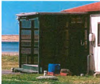
Whare Kai Porch: Bend in the drainage – and the clear cover was torn and dangerous.
