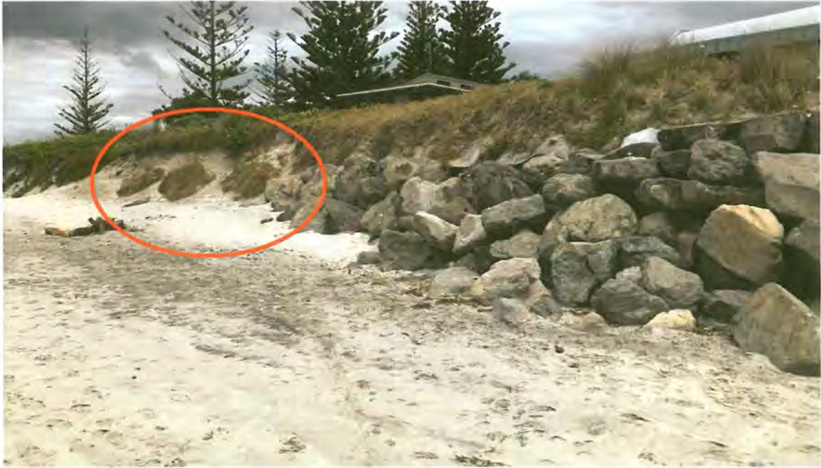
Figure 14b - Southern Termination of the Southern Seawall (red circle indicates more significant end effect erosion)
