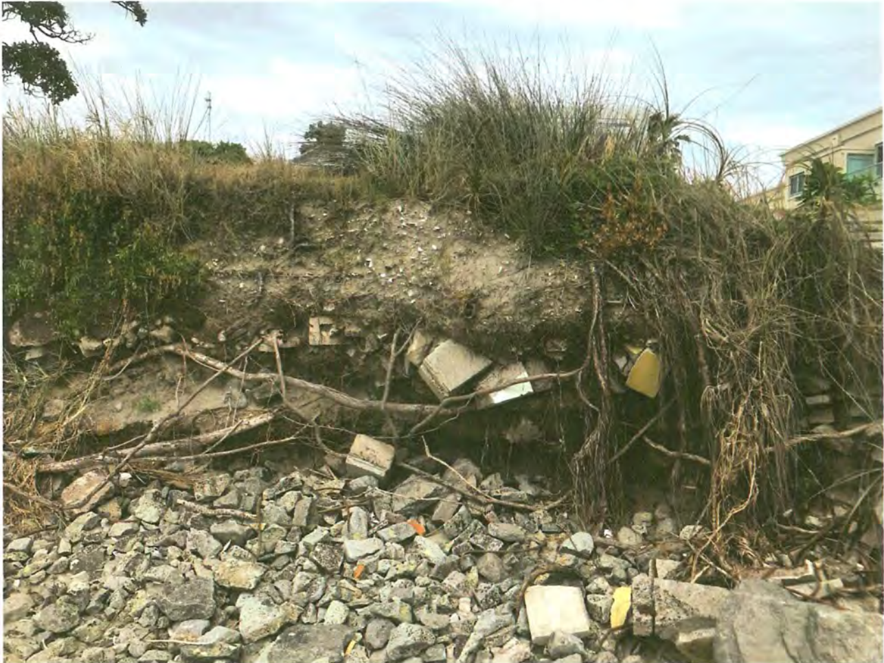
Figure 6 – Vertical bank littered with buried construction debris (Section A-A)
