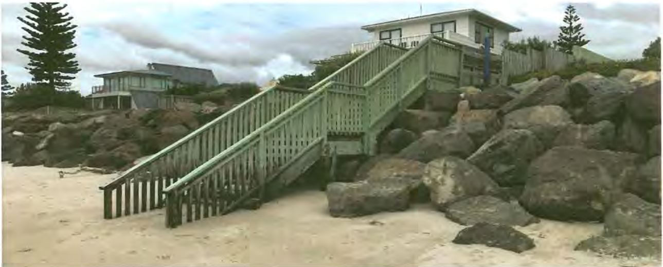
Figure 3 – Seawall showing accretion at seawall toe and a public access structure over the wall
