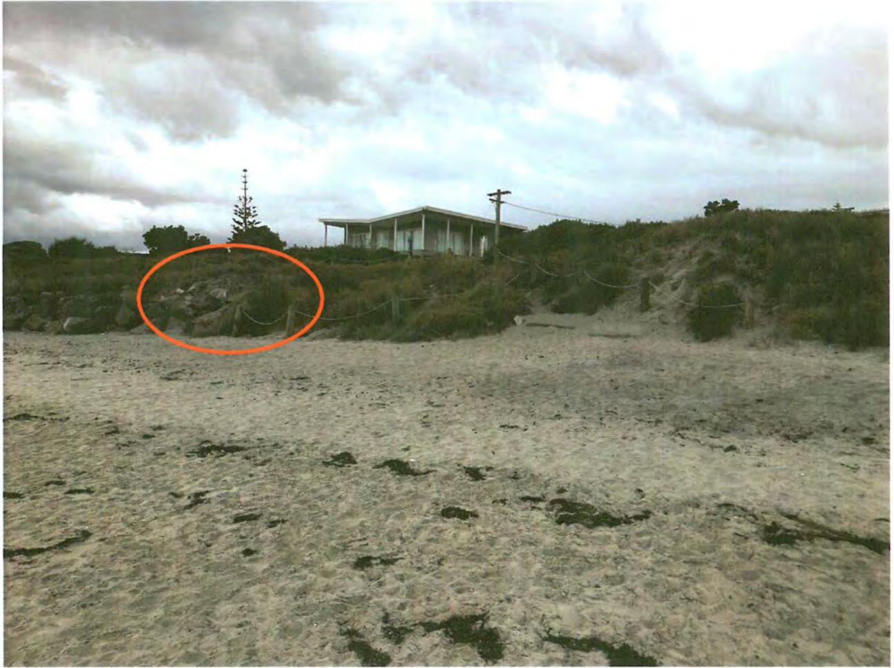
Figure 13a - Northern Termination of the Southern Seawall (red circle shows minor end effect erosion)
