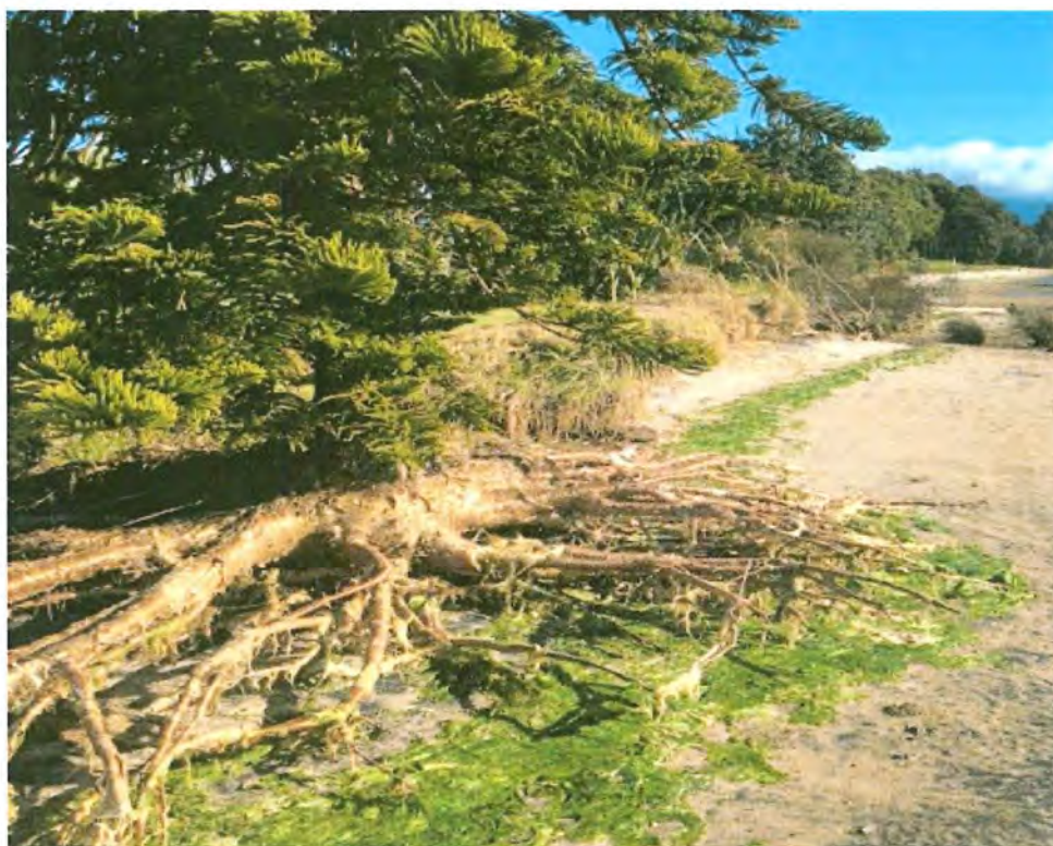
Typical erosion and retreat is shown in the photograph above.
