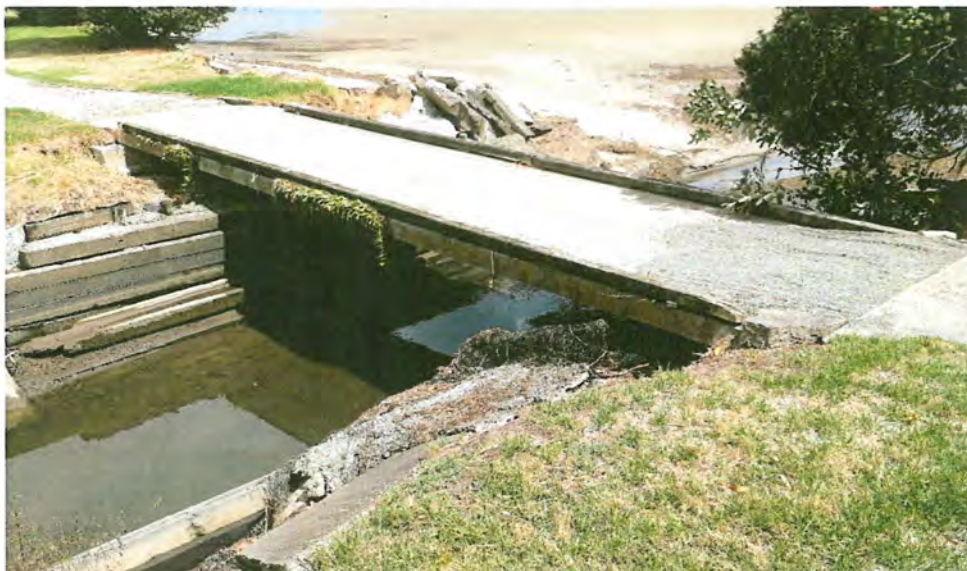
Typical ad hoc bridge solution:
