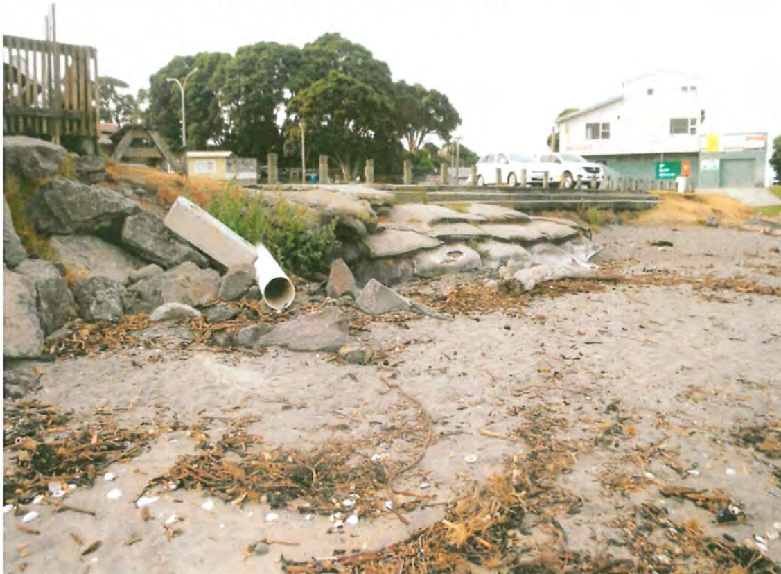
Car-park undermining & erosion processes – 18 February 2019.
