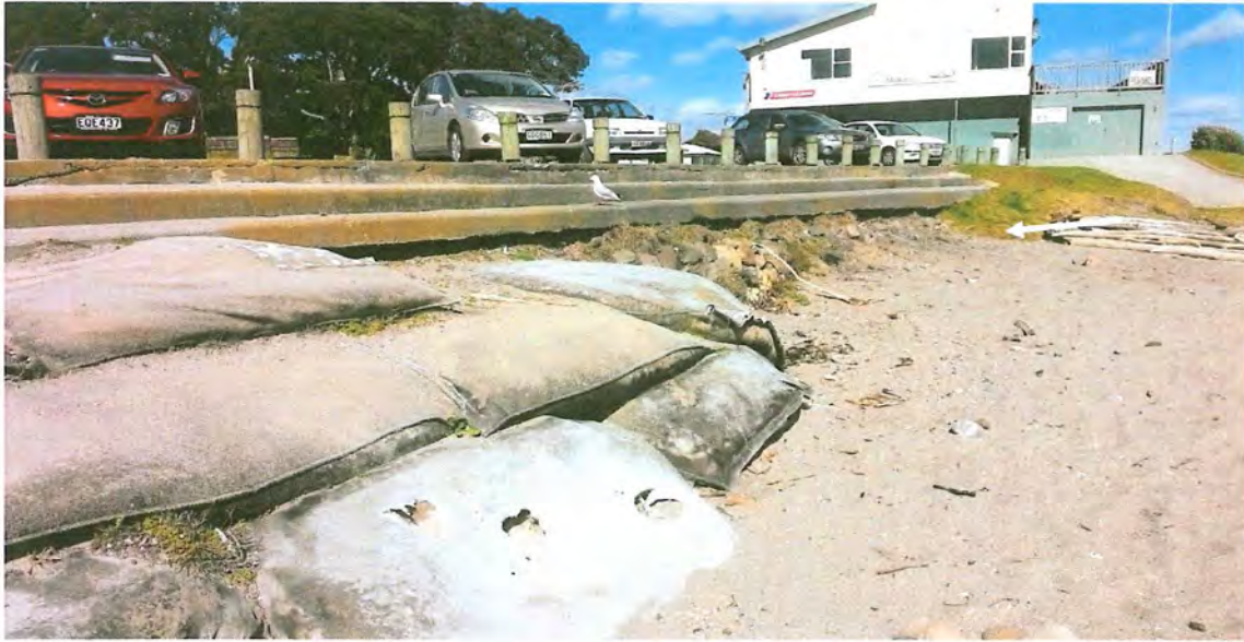
Car-park undermining & erosion processes – 2014.
