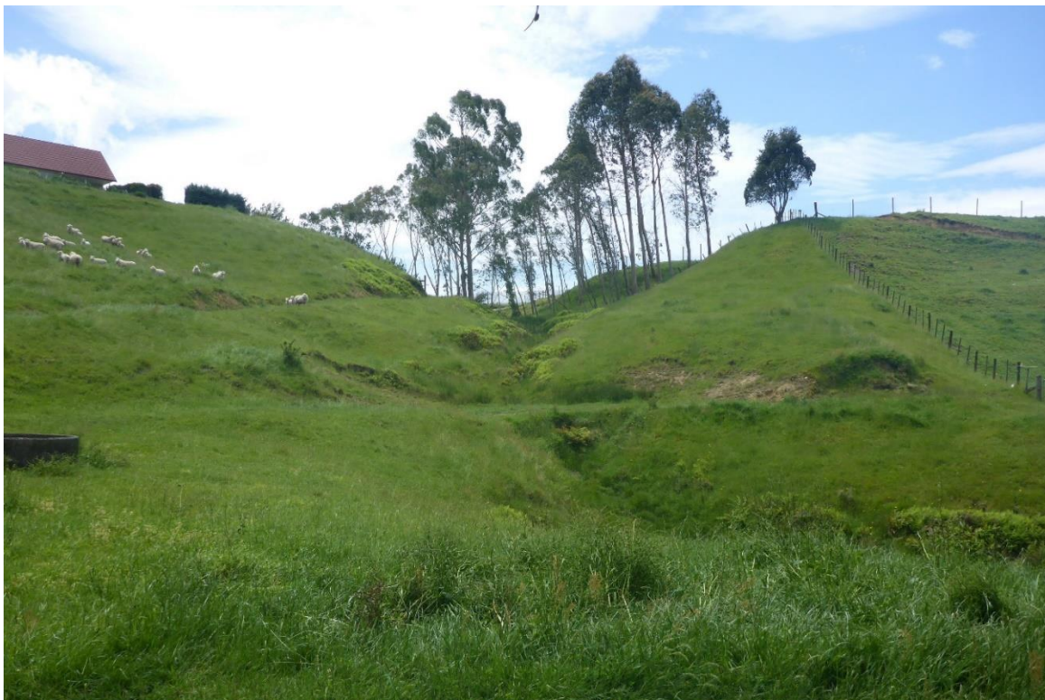
Figure 2-11: Reach Omo_E2 which has the highest erosion susceptibility. Note the steep slope, confined valley floor, access for stock, culvert, and evidence of bank erosion already occurring
