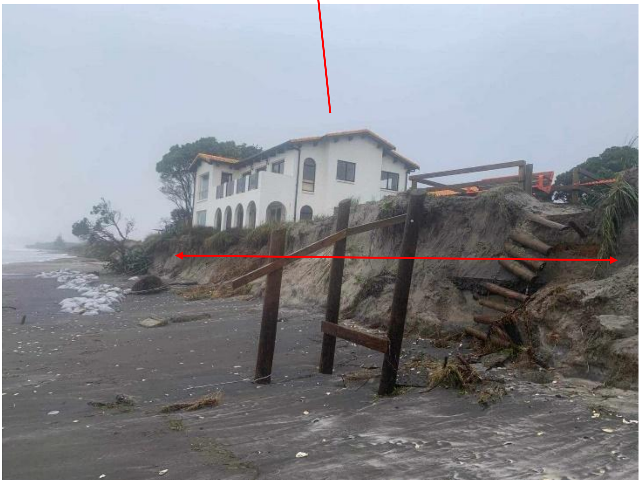
Figure 7 – Proximity of the erosion issues at 65 Broadway (successfully managed using dune repair - figures 5 and 6)
