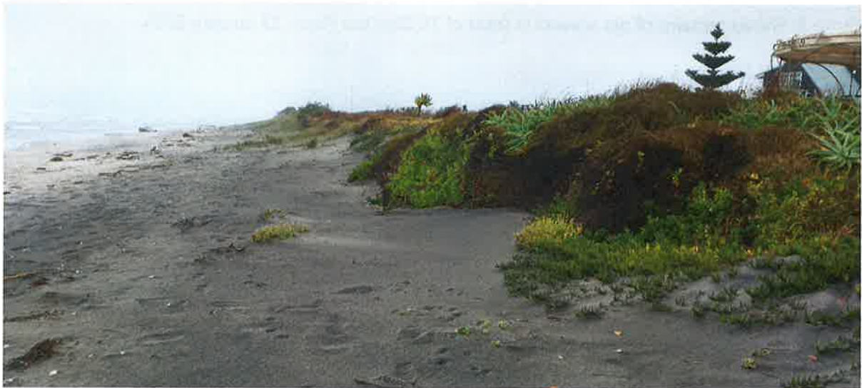
Photo 12: Shows Remains of old seawall in front of 16 Glen Isla Place 23 January 2025.
