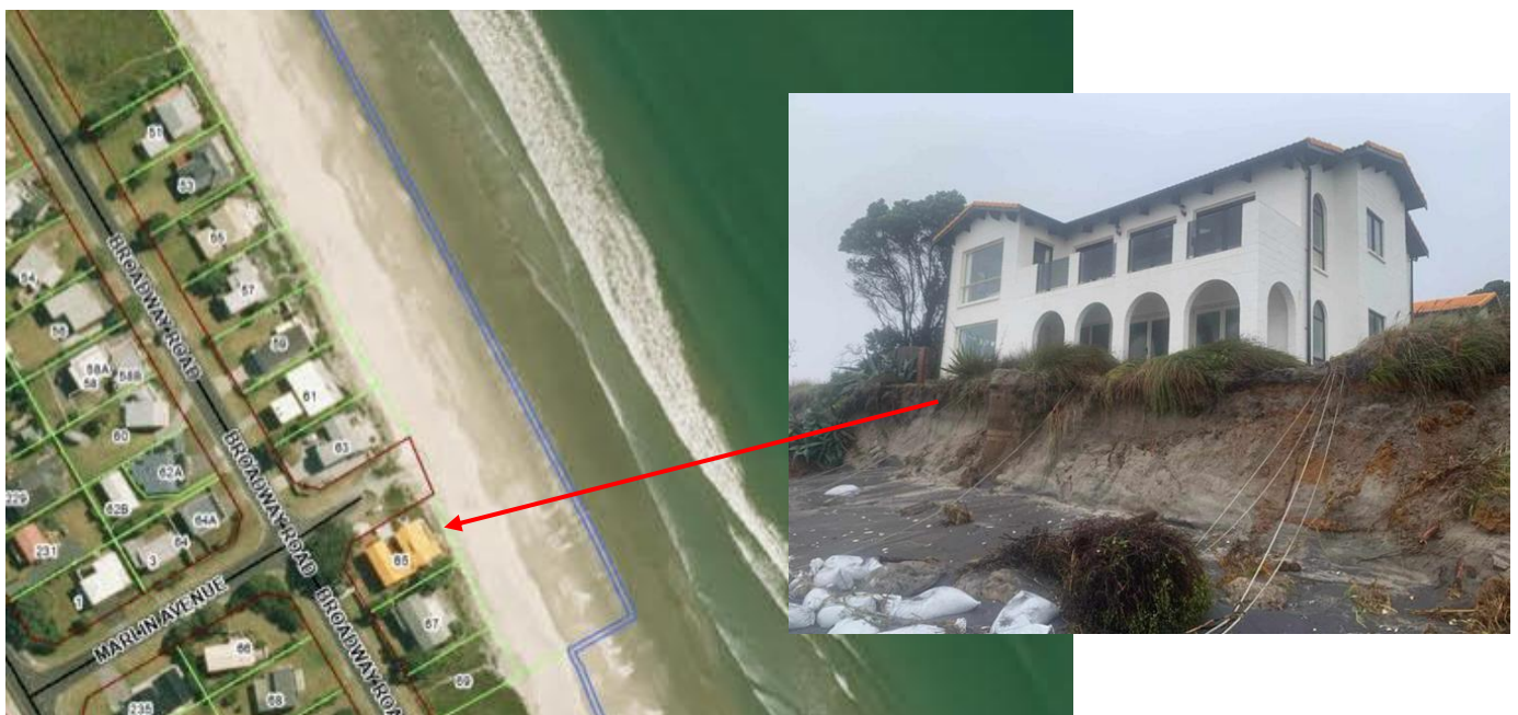
Figures 2 and 3 – Proximity of the erosion issues at Broadway. (later successfully managed using dune repair).
