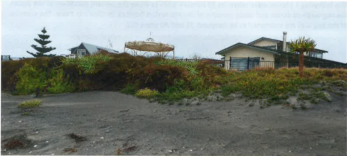
Photo 11: Shows Remains of old seawall in front of 16 Glen Isla Place 23 January 2025.
