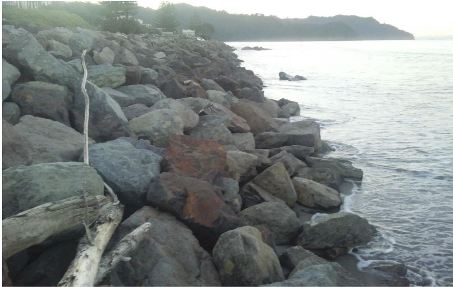
Figure 1: Examples of the seawall on The Loop and Shaw Road Waihi Beach showing the absence of beach at high tide.
