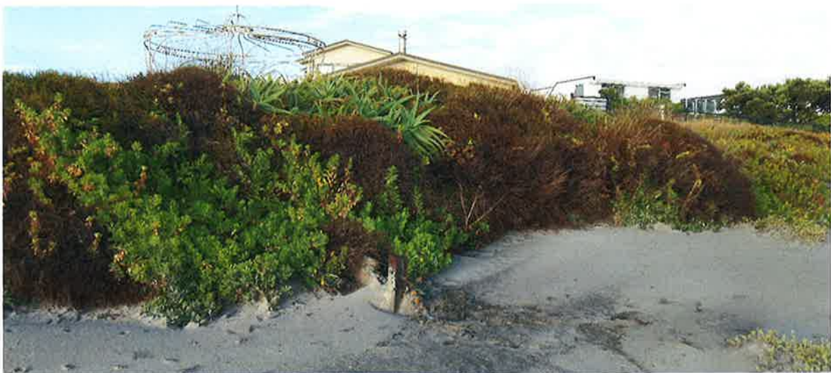
Photo 10: Shows remains of old seawall in front of 16 Glen Isla Place, 23 January 2025.
