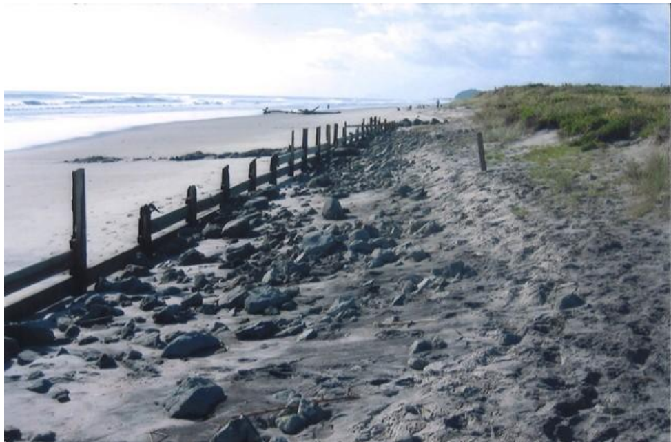
Image 2: The seawall constructed in 1983 with the sand level lowered after a storm, showing the gabion cages seaward of the wall and rocks behind the wall (date of photo unknown but between 1997 and 2011).
