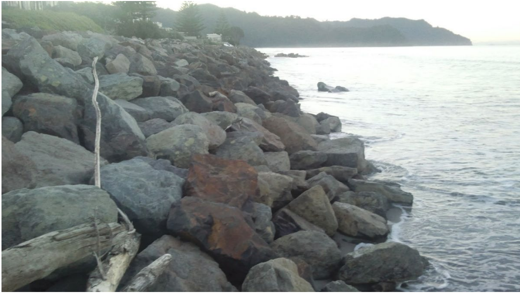
Figure 3: Seawall on Waihi Beach showing the absence of beach at high tide
