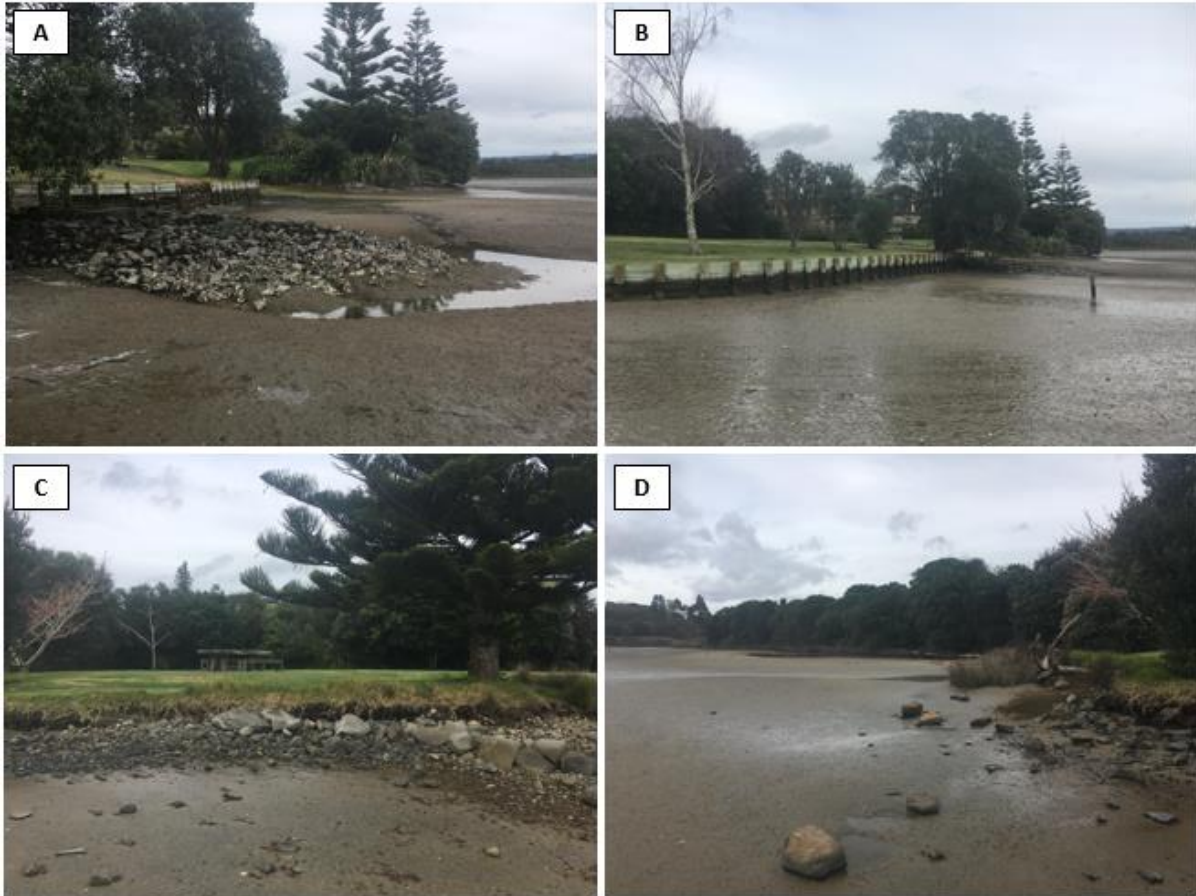
Figure 26-2 Site photos for Plummers Point West. (A) Rock around drain outfall (Cell 26D), (B) timber seawall (Cell 26D), (C) consolidated bank (Cell 26D), (D) low grass bank with patches of salt marsh (Cell 26E).
