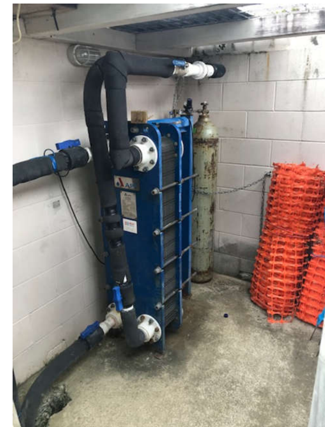
Toddlers Pool Heat Exchanger
