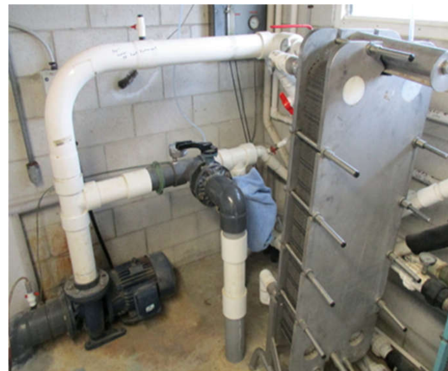
Main Pool Heat Exchanger
