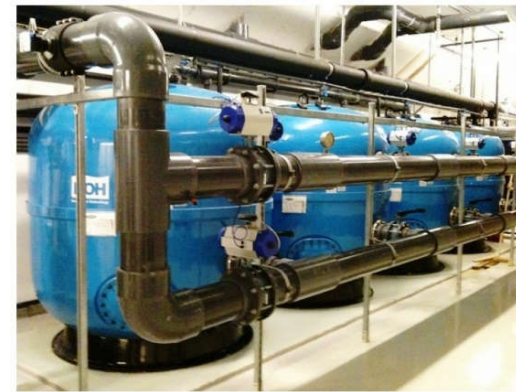
Pressure Sand Filters
