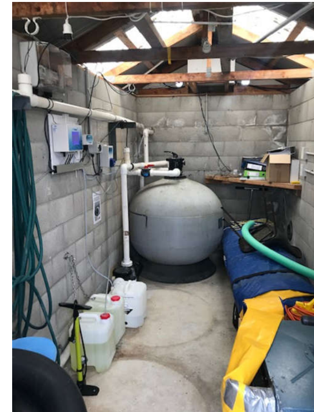
Toddlers pool filter and plant
