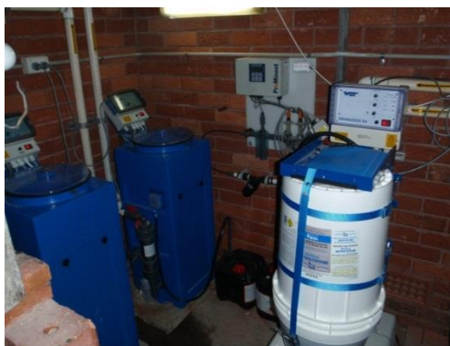
Chlorination system for three pools
